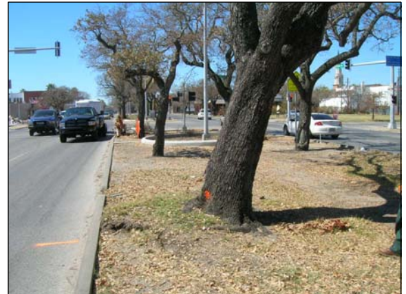
Live oak marked for removal due to root plate lifting
